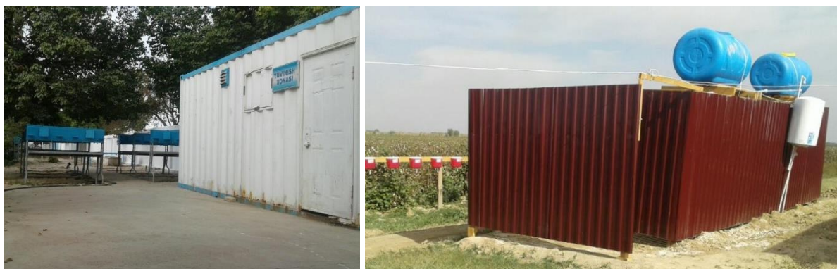
Pic 10. Hand washing facility – washstands.
